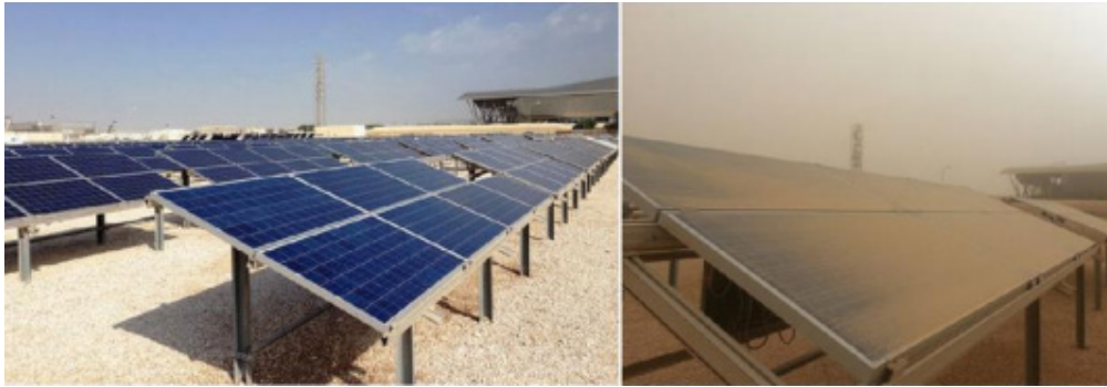
Figure 1. Solar panels before and after sandstorm accumulation
